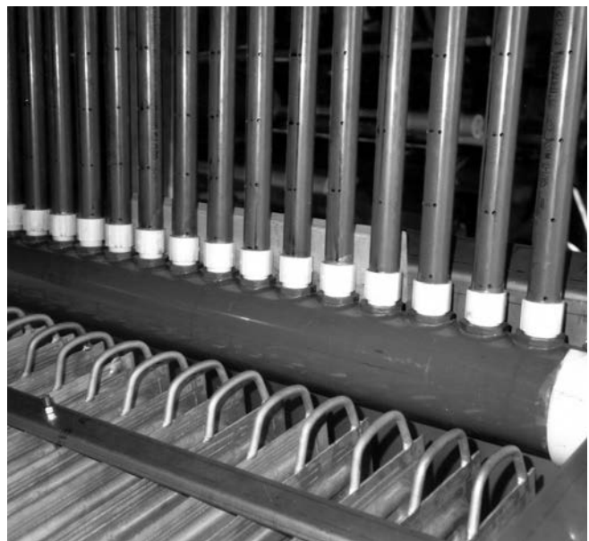
Fig. 56-2 These are Style 50D Serpentine PLATECOIL in a falling film chiller for a special anodizing operation.
